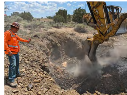
Runyan Construction excavating the burning coal at the Enterprise Brown fire. Temperature measurements were taken regularly to identify fire limits.
