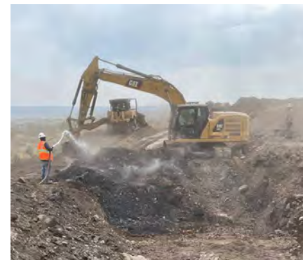
Runyan Construction excavating the burning coal at the Navajo No.1 fire. Water trucks were used to cool the temperature of the piles and suppress excess dust.
