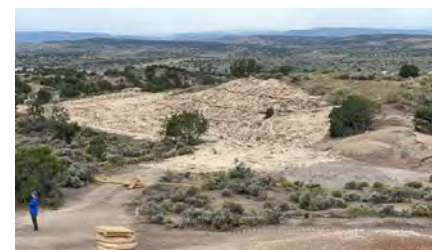
Post-fire mitigation reclamation work at the Navajo No. 1 site. Wood mulch was applied over native seed.
