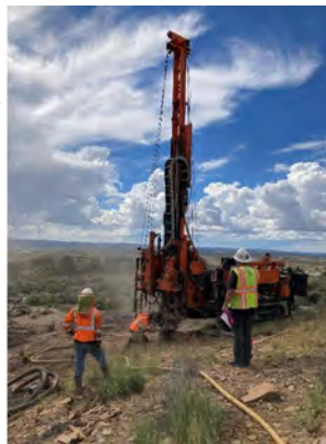
Geotechnical drilling (Authentic Drilling) to determine the extent of the coal fires.
