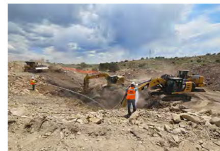
Heavy machinery used to extinguish the coal fire at the Enterprise Brown mine.
